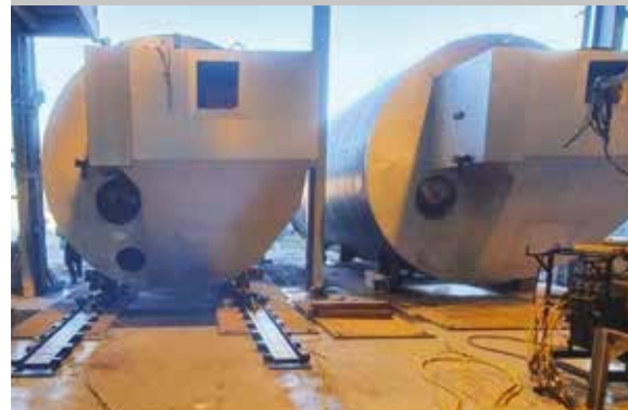
The boilers safely outside the boiler house.
